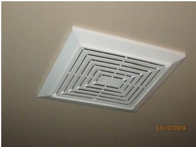
Close up view of soffit mounted bathroom exhaust fan.
