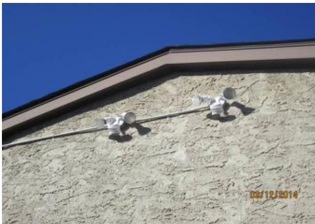
Typical wall mounted building light fixtures with motion sensors observed at Block 6.
