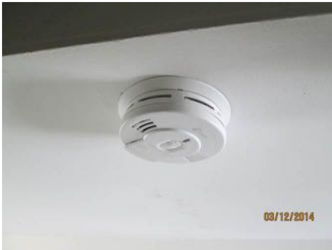
Typical battery operated smoke alarm observed in working condition.
