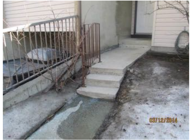
Metal guardrails on top of retaining wall & concrete entry steps at Block 4 observed.
