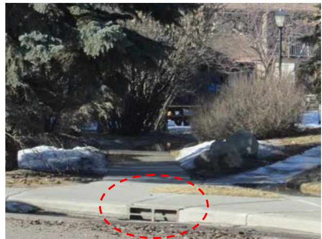
Typical storm sewer system throughout the property.
