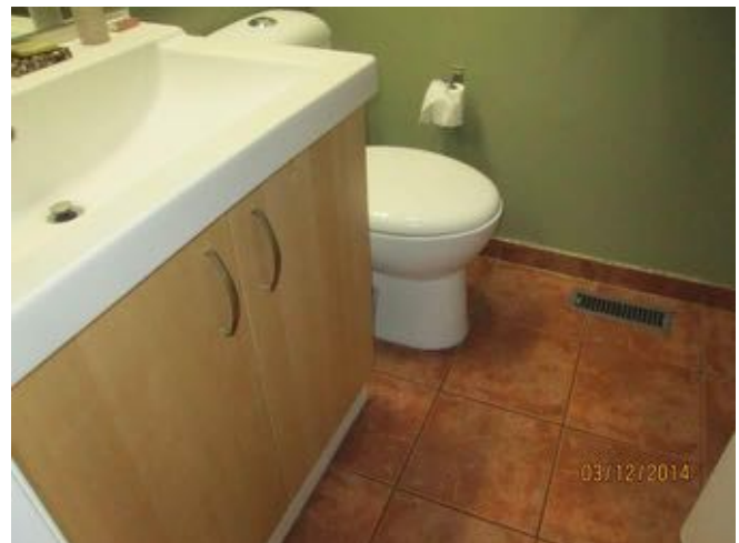
Ceramic floor tiling observed in the bathroom of a townhouse at Block 2.
