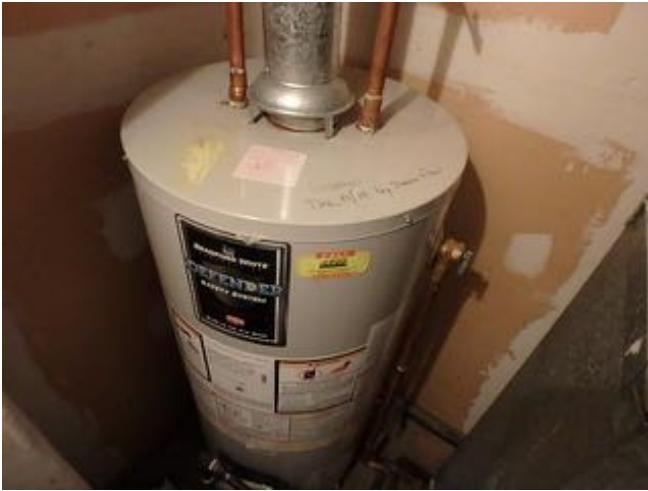
Typical Bradford White Hot water storage tank.
