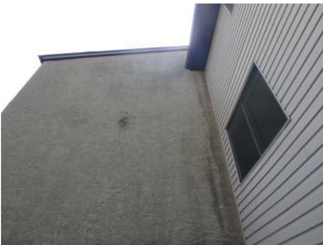
Water staining noted on end wall areas under eaves troughs
