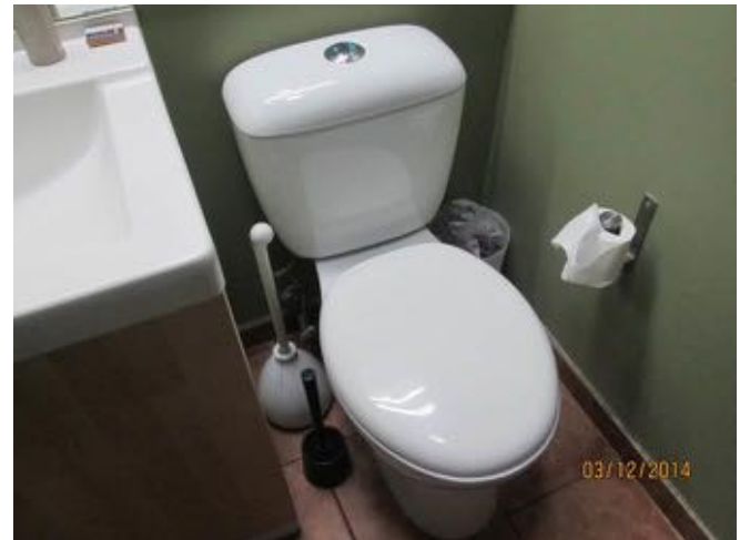
Typical dual flush type toilet observed in a townhouse unit.
