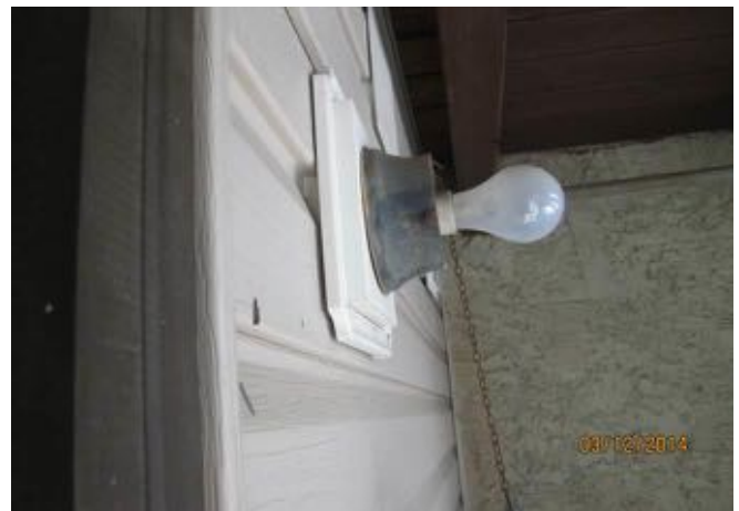
Typical incandescent light fixture at Unit 42 observed.
