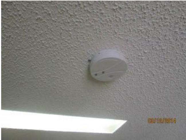
Battery operated Kidde smoke alarm in the Sunnyhill Co-op's office at Block 2.
