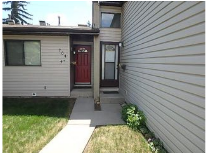
Concrete steps & walkways with localized cracks.
