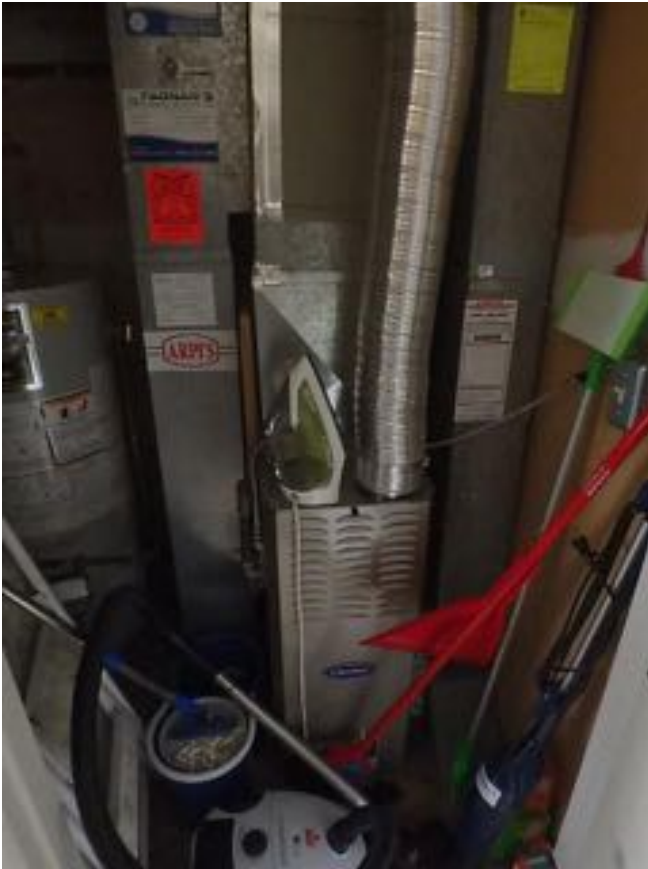
Typical gas-fired Carrier furnace observed at the 2 nd floor level of the townhouse unit.
