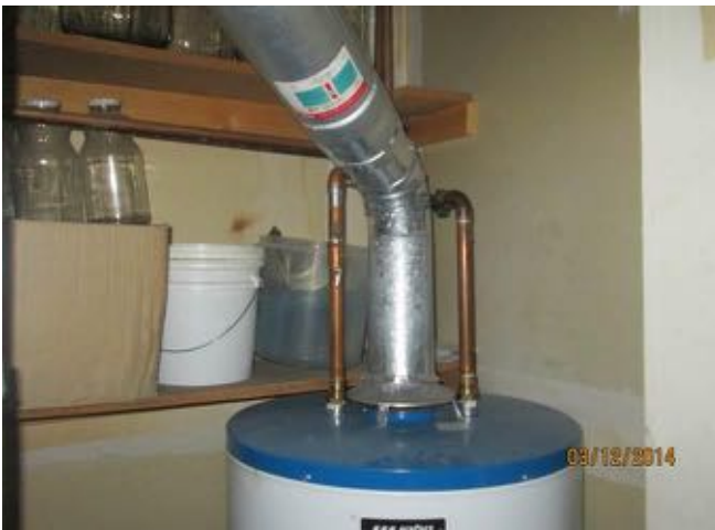
Typical copper pipe connection to an automatic storage water tank.
