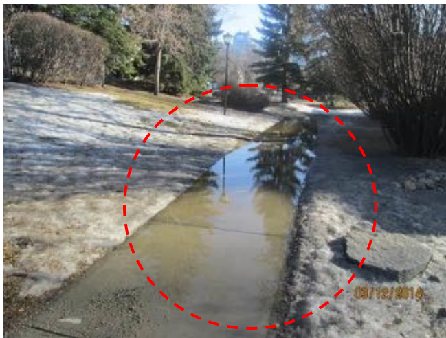
Ponding water observed at the concrete walkway between Blocks 6 & 7.
