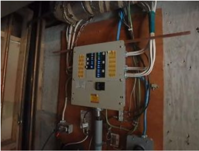
Typical circuit breaker in the townhouse unit reviewed.
