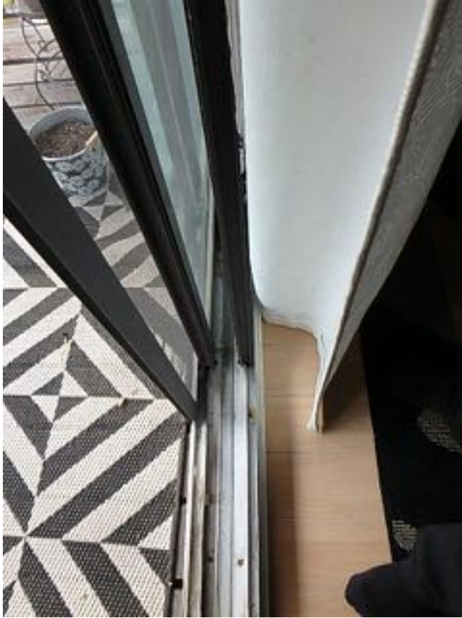
Typical sediment build-up and glider wear on balcony sliding door track
