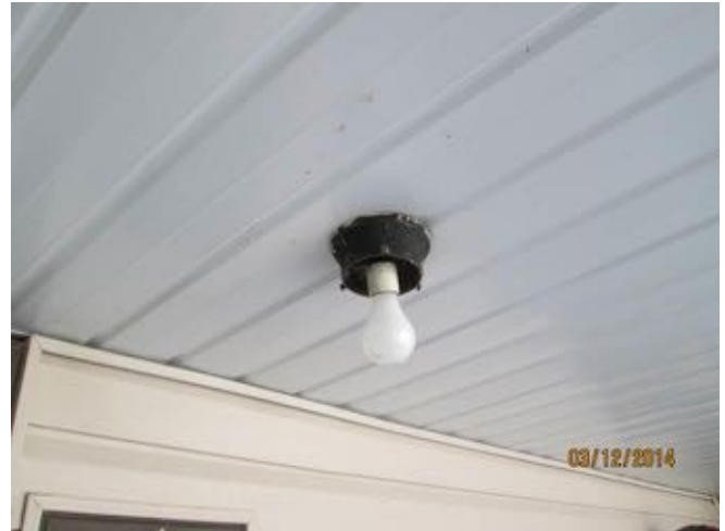
Soffit mounted incandescent light fixture observed at unit 22.
