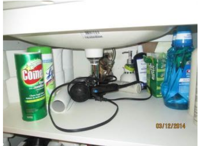
Typical piping layout servicing a bathroom wash basin.
