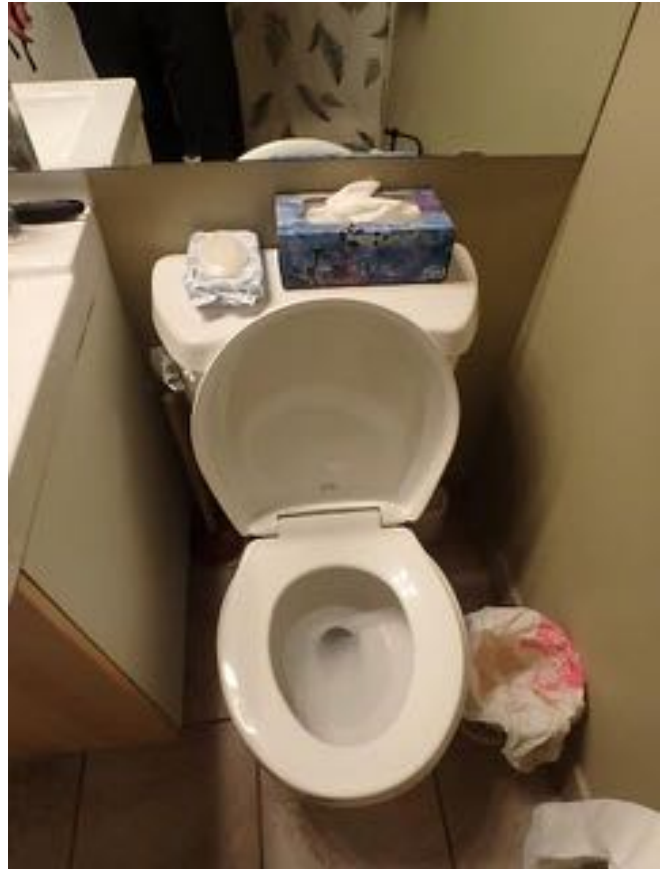
Typical upgraded low flow toilet.
