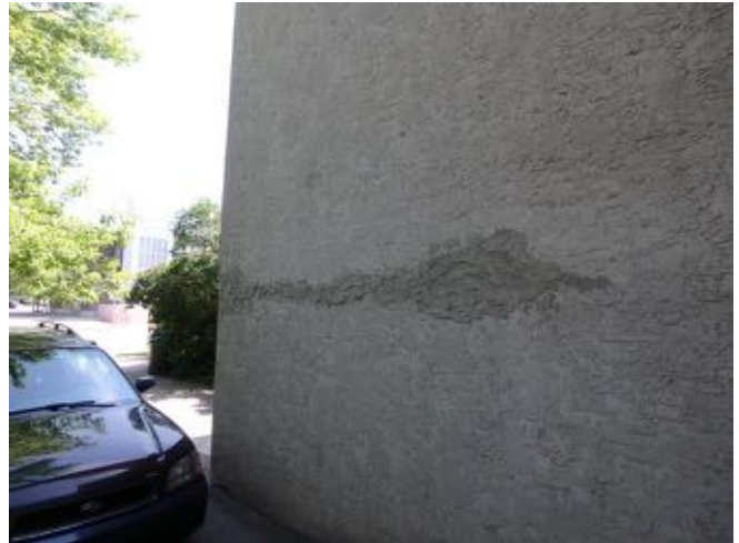
Evidence of historic parking repairs noted on concrete foundation.
