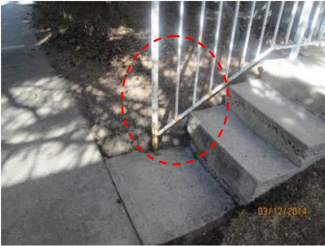
Metal guardrail exhibit corrosion at a townhouse unit entry steps.
