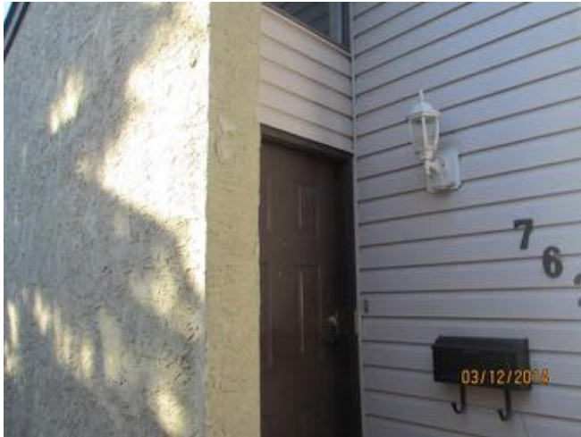
Typical wall mounted light fixture at unit 762 observed.
