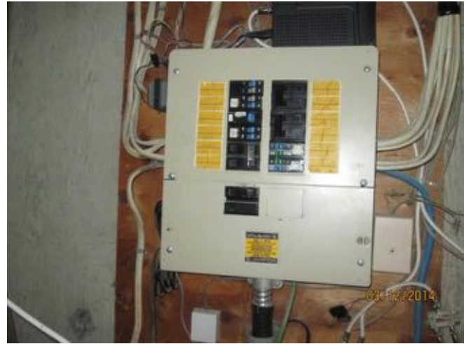
Typical NOVA Line NLC 24 circuit breaker observed.
