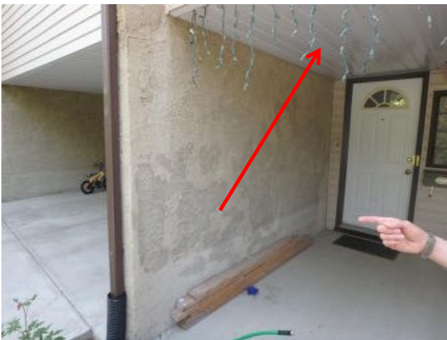
Typical pre-finished aluminum soffit at the main entrance & carport area of a townhouse
