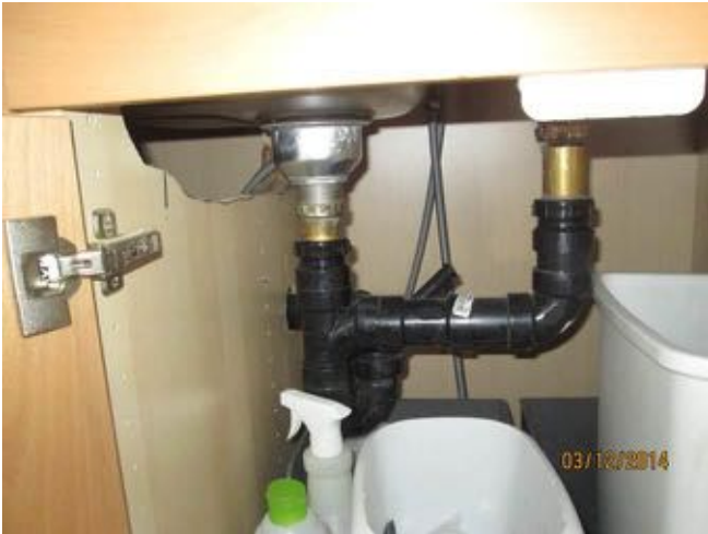
Typical piping layout servicing a kitchen sink.
