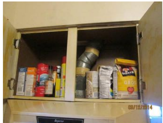
Typical kitchen range hood and ducting observed at a townhouse unit.
