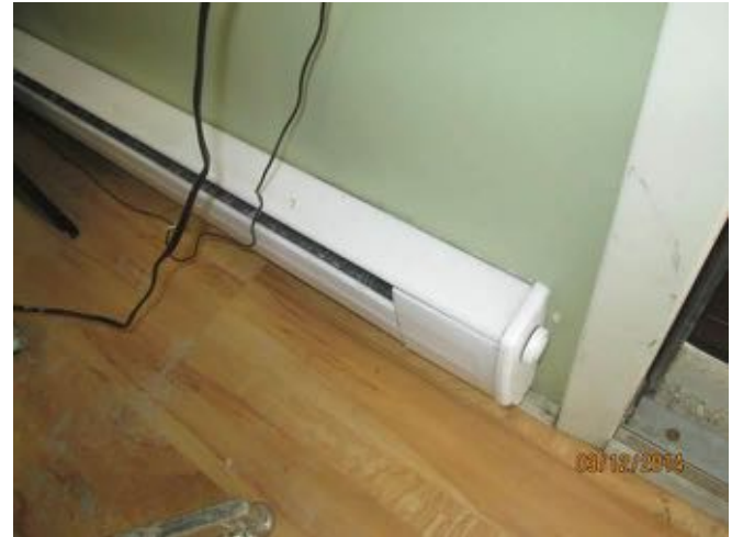
Electric baseboard heater in the office at Block 2 observed.
