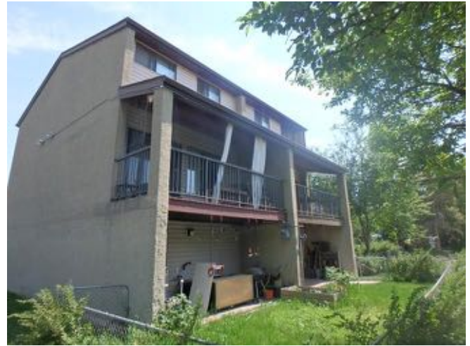
Typical water staining and moisture damage on stucco at balcony to end wall locations
