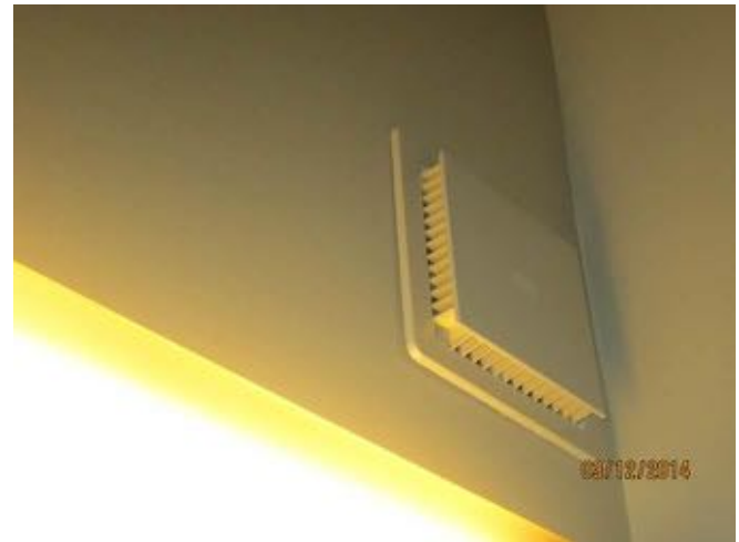
Typical wall mounted bathroom exhaust fan observed in working condition.
