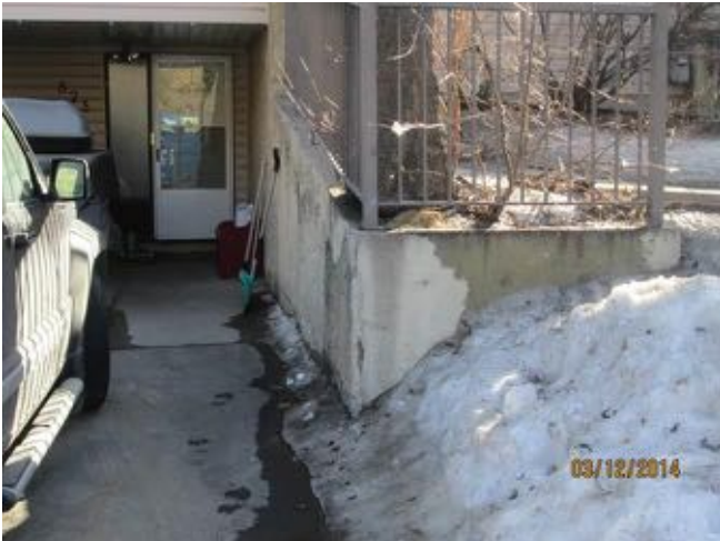
Close up view of metal guardrail on top retaining wall at Block 4.
