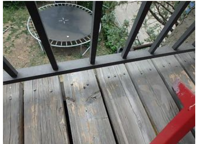
Unsecured/backed out nails observed at the balcony wood planks & cracked & minor rot at townhouse unit 811 of Block 2.
