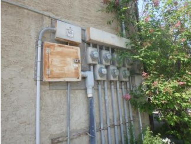
Typical electric meters & electrical panel observed.
