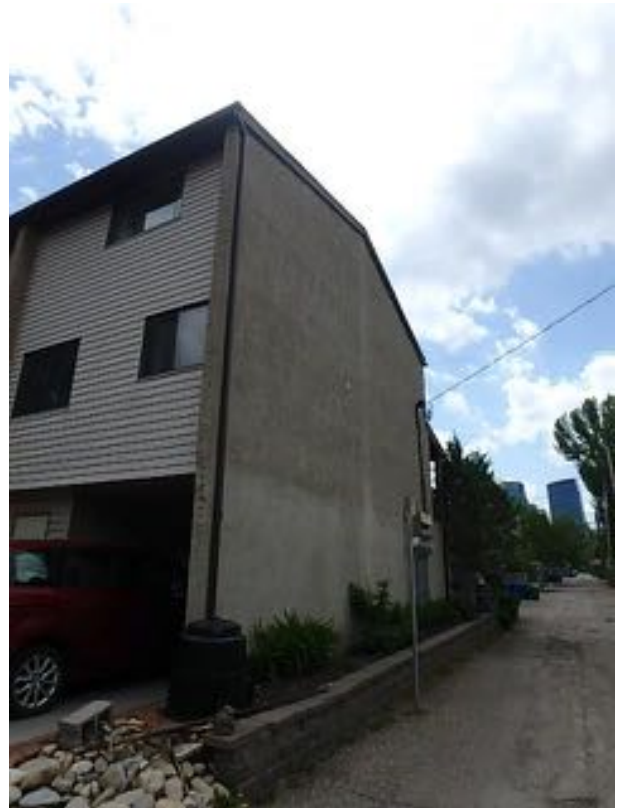
Typical patch repairs at end wall areas at concrete to wood frame transitions.
