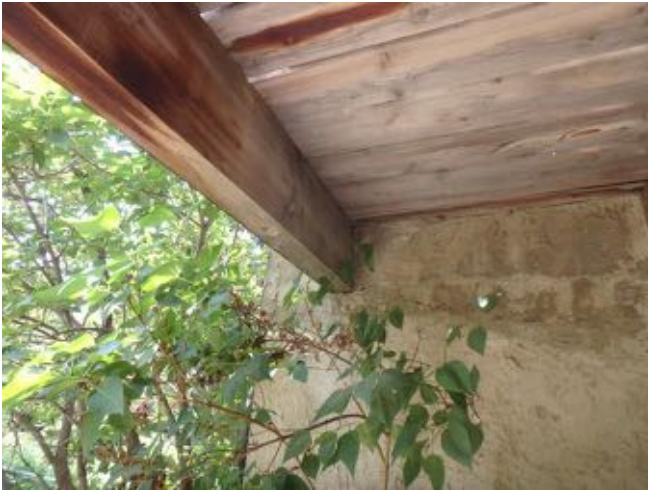
Typical water staining on stucco under balcony areas.
