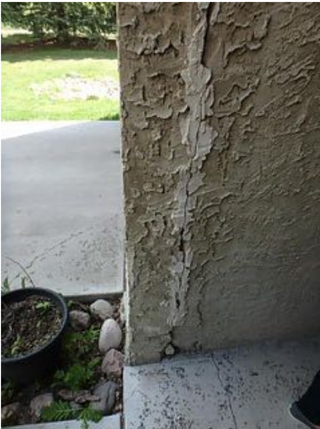
Isolated delaminated concrete section.
