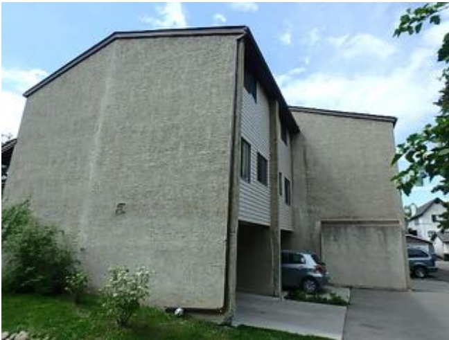
Damaged Stucco located at end wall for unit 44 (or block 8).
