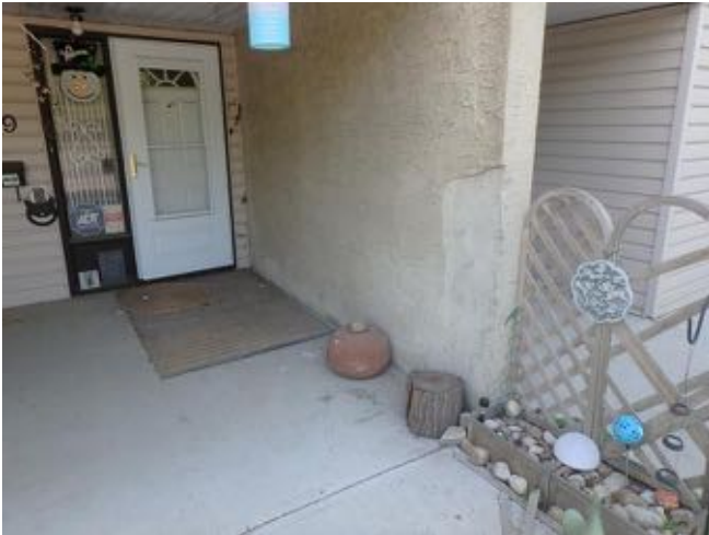
Parging noted to be delaminating from Concrete foundation (non-structural concern).
