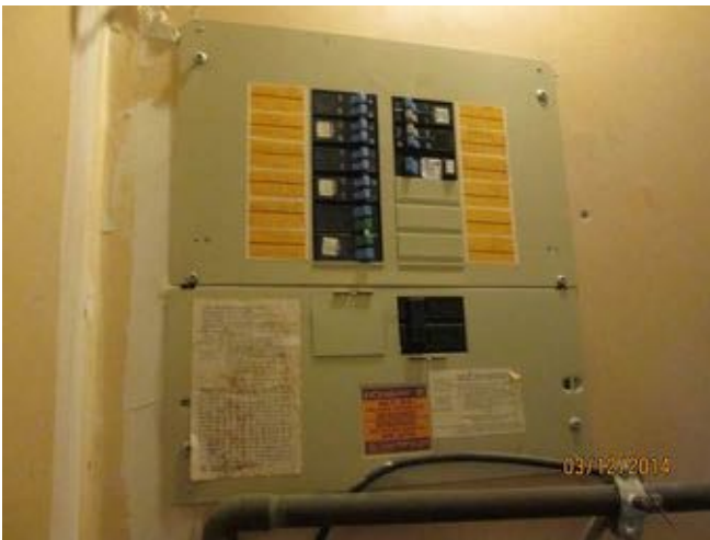
Typical surface mounted Westinghouse NOVA Line circuit breaker observed.
