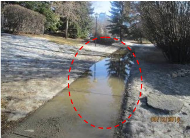
Ponding water on concrete walkway observed between Blocks 6 & 7.
