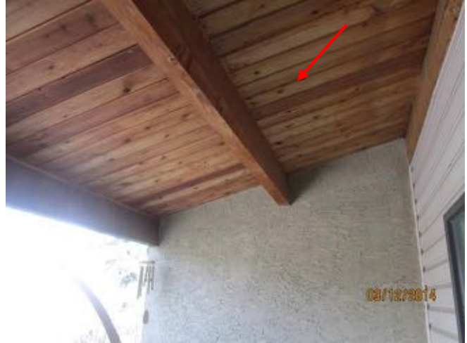
Typical tongue & groove cedar wood soffit above the townhouse unit balcony observed.
