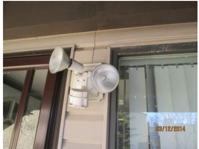
Wall mounted light fixture at with motion sensor observed at the common office at Block 2 observed.
