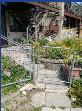
Figure 5: Problematic office entrance
