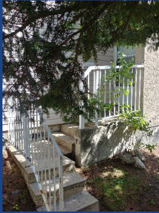
Figure 7: Staircase non-compliant to current building code
